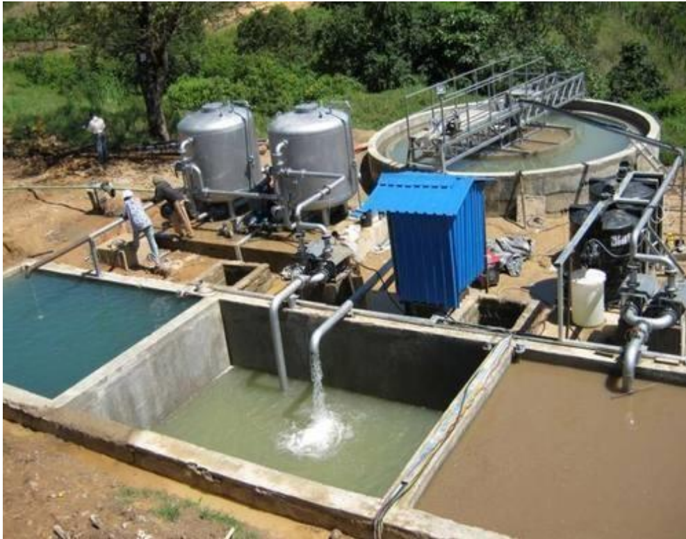
Fig 3., Effluent treatment plant
